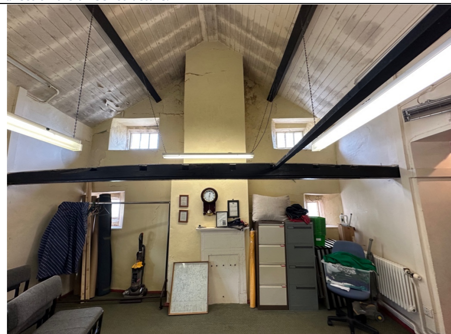
073 – General of the first floor meeting room looking toward the North East gable end wall.
