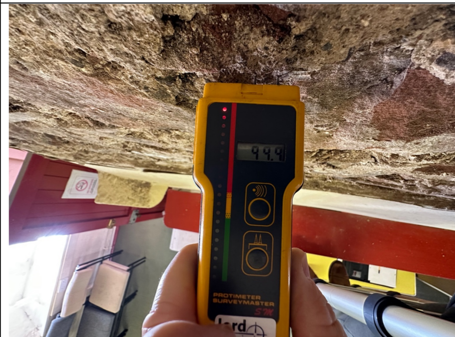
060 - Exposed masonry to the chimney breast structure identified in photo 056. In this location (chimney breast) the Protimeter presented moisture levels of 99.9%. Indicating almost full saturation of the structure.
