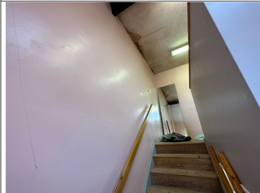
049 – View from the ground floor of the store room looking up to the upper first floor level. Note: the heavy water staining and discolouration of the ceiling at first floor level.
