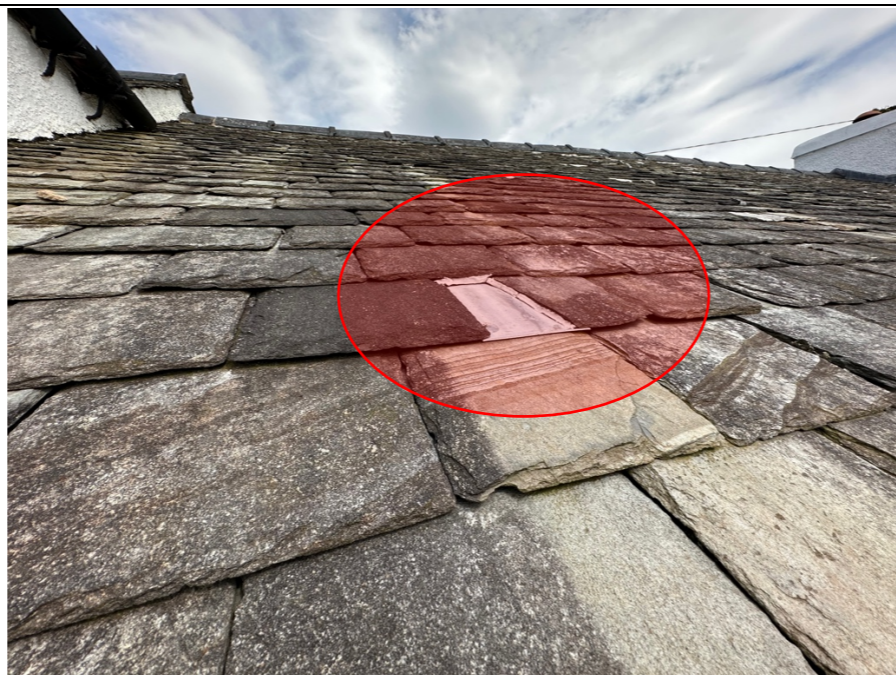
013 – Evidence of a non-typical slate repair to the rear addition roof covering.
