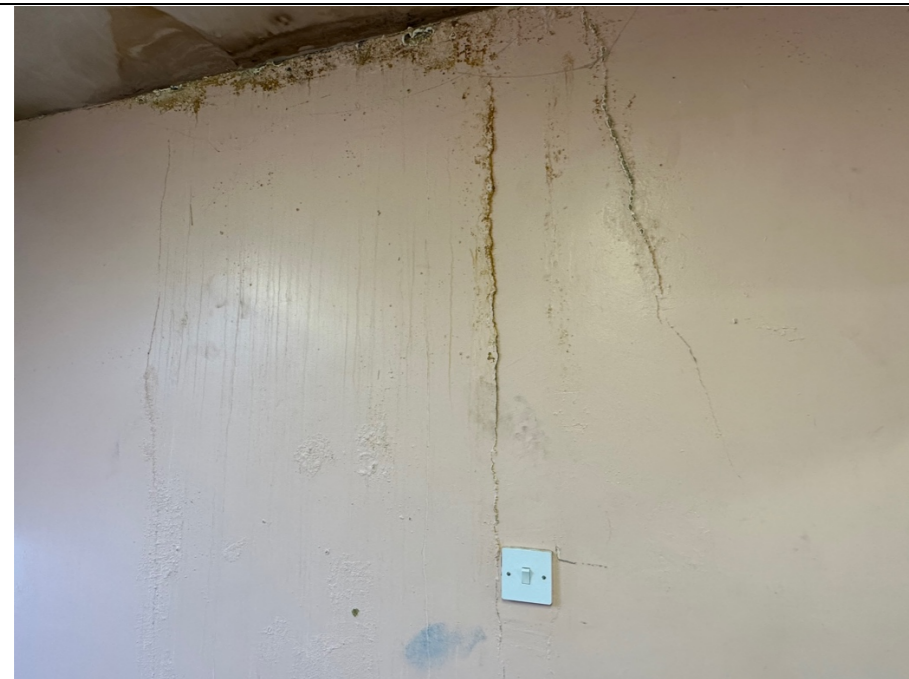
055 - Image of the recently plastered ceiling area above the staircase. Note: Further investigation required, which may entail destructive works to expose the potential ingress point and to also inform on the condition of the timber roof structure, which will have been exposed to penetrating water for some time.
