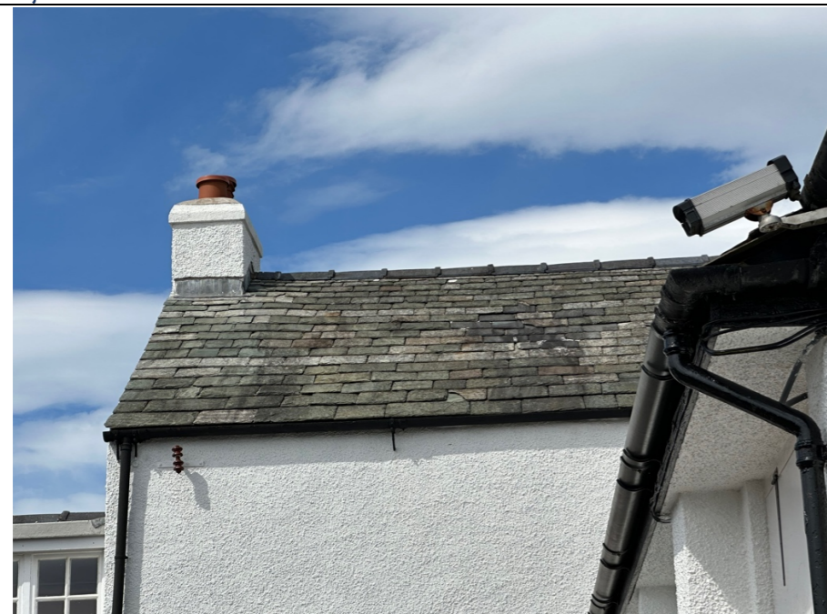
007 – South East facing slated pitched roof slope of the traditional Grade II Listed building.
