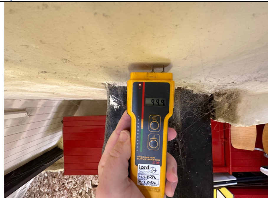
070 – Intermediate principal timber roof truss to the roof structure above the meeting hall. Truss is bearing into the principal front elevation wall.
