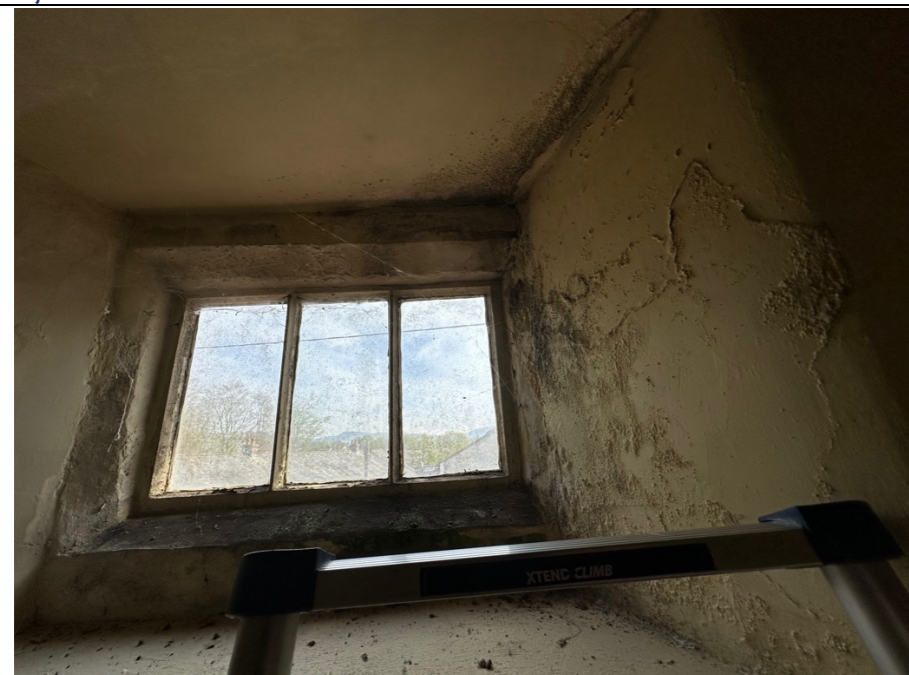
076 – High level window identified in photo 074. Extensive disruption of the painted and plastered wall surfaces as well as to the sandstone window surround. Evidence of algae growth to sandstone and mould growth.
