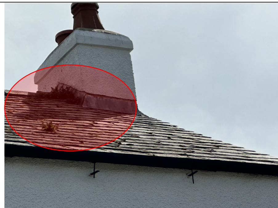
005 - Evidence of not just general moss growth to the pitched roof slated surface to the front elevation, but also of actual vegetation growing from beneath and between the slate roof covering. Indicated sufficient presence of damp to maintain vegetation growth. North West orientation.
