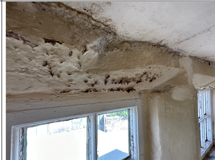
069 – Sandstone lintel above a meeting room timber framed window on principal elevation. Extensive flaking and general deterioration in the painted surface of the natural stone lintel. Evidence of water staining to surrounding finishes, related to the trapped moisture behind the external rendered wall finishes.
