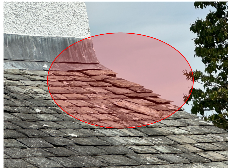
010 – Slating to verge on the North East gable elevation (SE facing roof slope). Slates are lifted and misaligned. There is evidence to suggest that the loose slate resting on the slope has in the past been stuck down with some form of mastic sealant.
