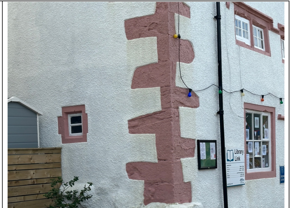
028 – North East facing gable end wall concentrating on the external corner of the building and the quoin stone detailing. Note: The general discolouration of the render finishes around the quoins.
