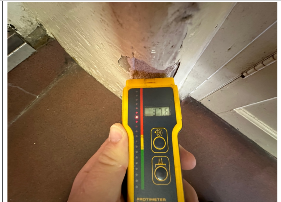
033 – Around the building a Protimeter was used to record the condition of walls and partitions in respect of moisture / damp. Readings were taken using the two pins of the Protimeter penetrating the surface of the wall / partition.
