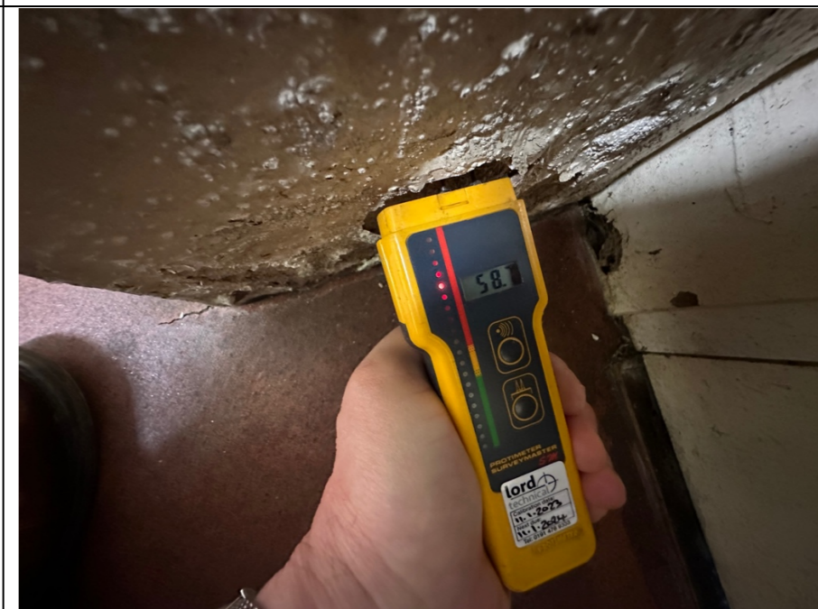
039 - In this location (adjacent to the external door) the Protimeter presented moisture levels of 58.7%. Which indicates there are issues with rising damp to the lower areas of the wall in this location and equally are possibly associated with the external render issues identified earlier..
