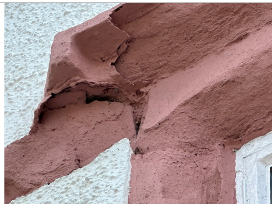
021 – The extent of deterioration to the natural stone moulding is believed to be beyond repair, as too much of the material has been lost. Repair would always be the first option to consider when dealing with Listed and historical buildings as the premiss is always wherever possible to conserve the original fabric of the building.
