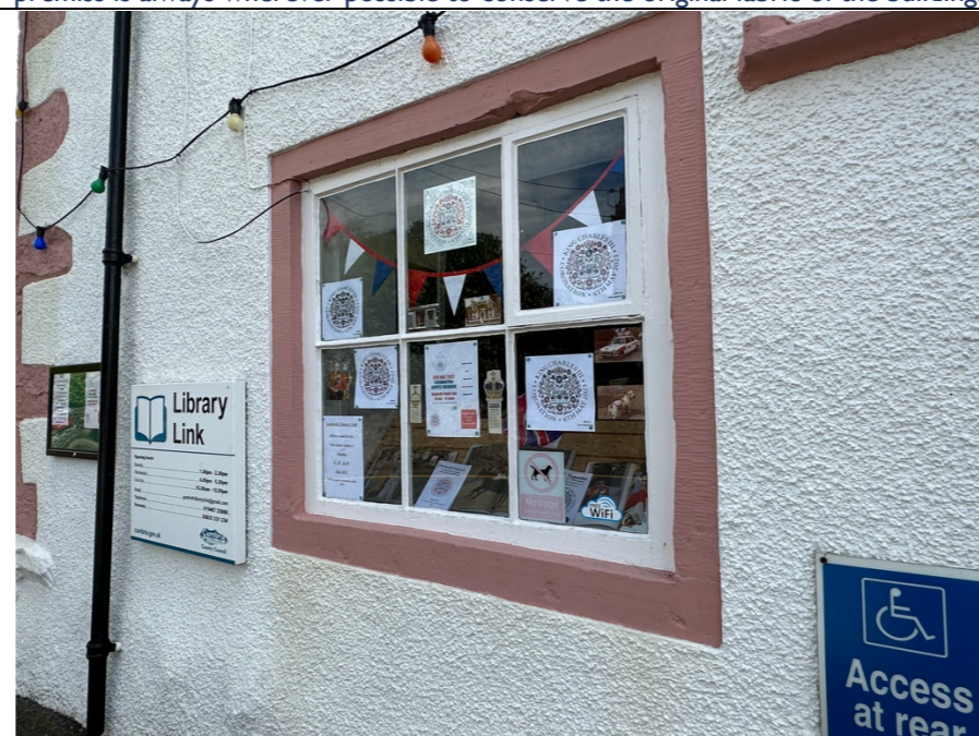
024 – Example of where the rough cast render finish has been built / up and applied to stand proud of the original sandstone detailing.
