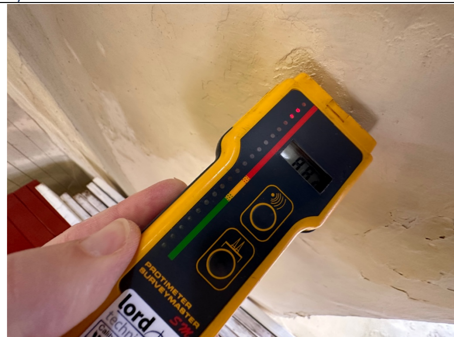
064 – Image of the principal front elevation to the left hand side of window 01 along the elevation (LHS) Extensive discolouration and staining to the internal plastered wall finishes. In this location (front wall panel) the Protimeter presented moisture levels of 88.2%.
