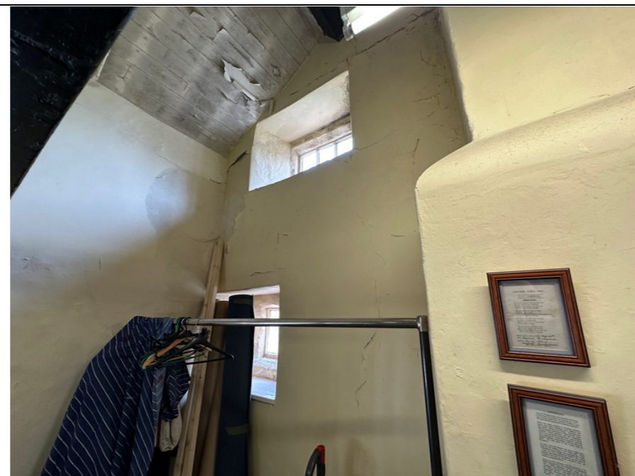
074 – General deterioration of wall finishes and boarded ceiling finishes to the left hand side of the chimney structure, spreading across to the principal front elevation.
