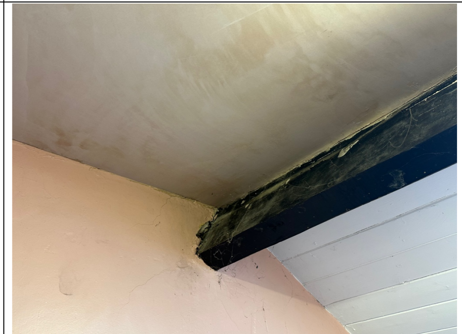
051 – Image of the recently plastered ceiling area to the left hand side of the rooflight. Note: There is a discolouration and unevenness to the new plaster, indicative of the area retaining moisture and suggesting any repairs undertaken to resolve water ingressions have not been entirely successful.
