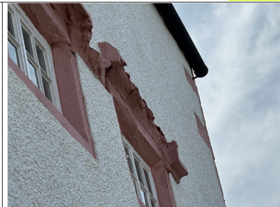
022 – Image of the window opening and detailing identified in image 020, it is clear that more than 50% of the original fabric of the cloaked moulding has been lost and that which remains is in a deteriorating and friable condition.
