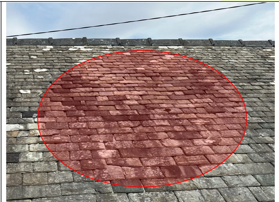
009 – General gapping of joints to the slate roof covering and within the 'red zone' the slates are showing signs of deterioration, including – gapping, broken & missing slates.
