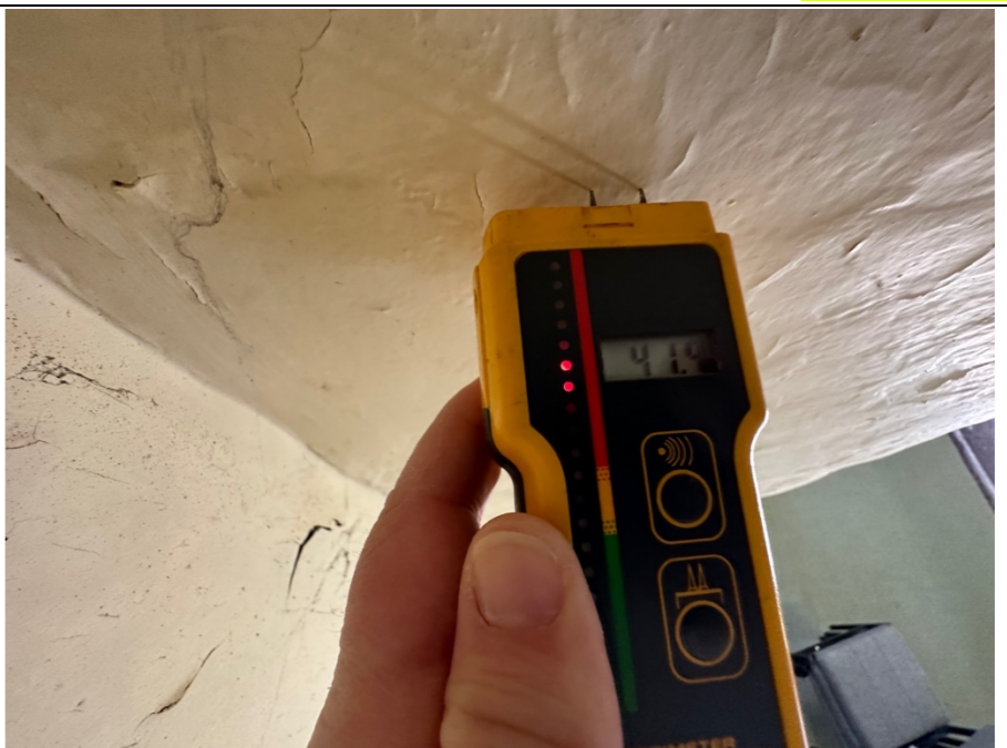
078 – Left hand reveal to the chimney breast structure identified in photo 073. In this location the Protimeter presented moisture levels of 41.4%.
