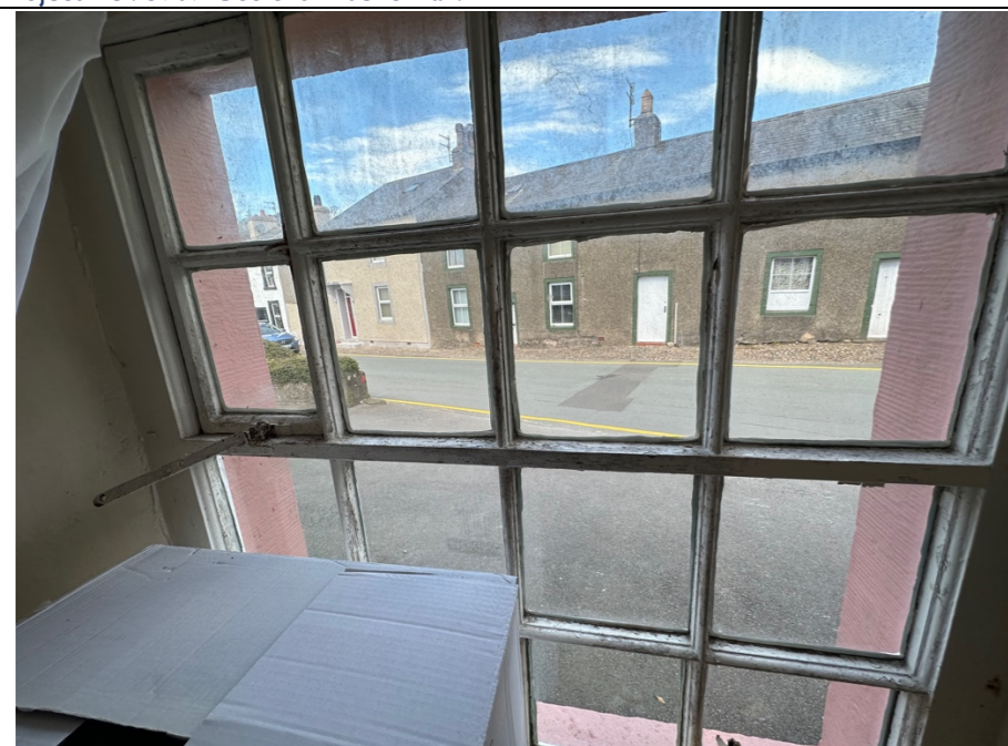
040 – Kitchen window within the principal elevation external wall. Whilst decorated externally, the internal condition of the decorations to the timber joinery is in a deteriorating condition.
