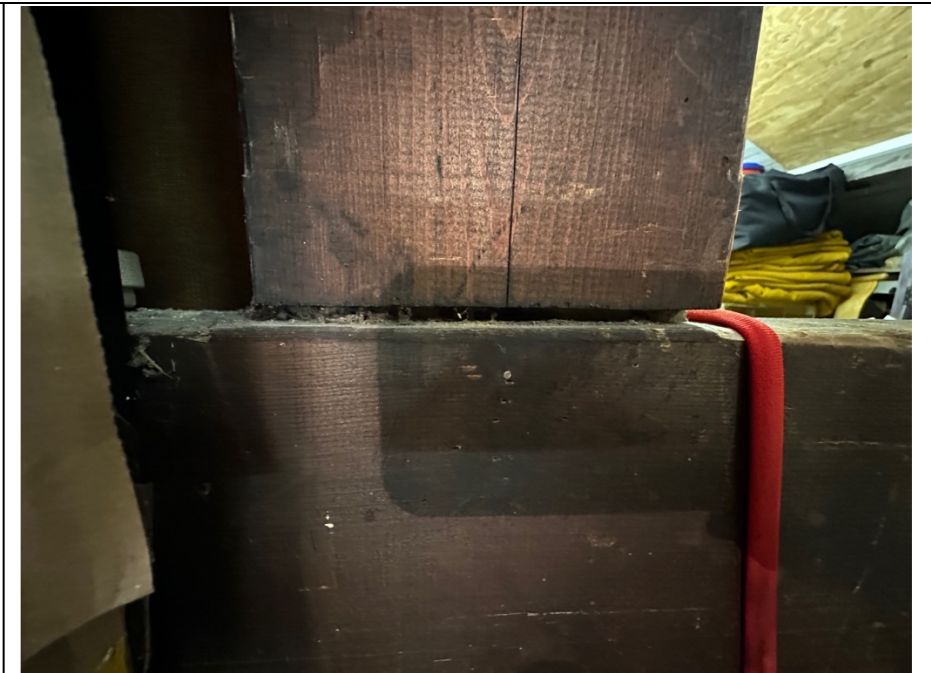
084 – A consequence of the additional loads imposed on the timber truss sections is that the joints between the truss members are being forced to part.
