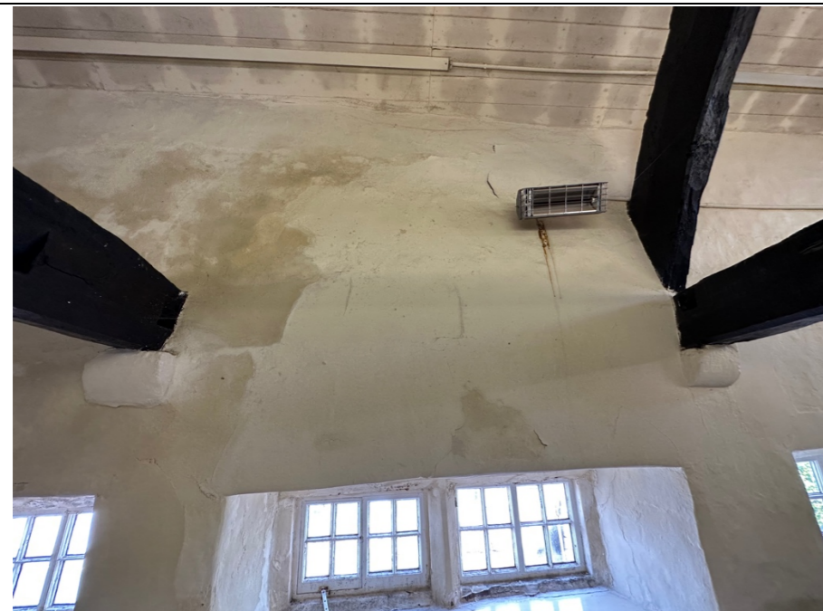
067 - View of the principal front elevation to the traditionally constructed Listed building. There is extensive discolouration and staining to the internal plastered wall finishes, across the face of the wall.
