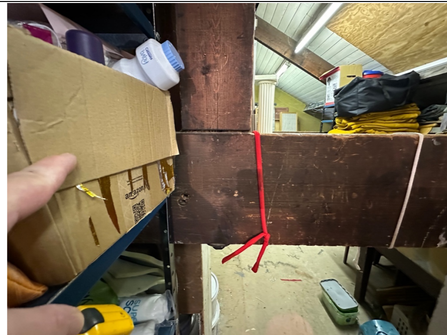
083 – Within the storage area, racking and shelving has been employed which in either part or wholly relies on the timber roof trusses that support the loads from the roof structure above.
