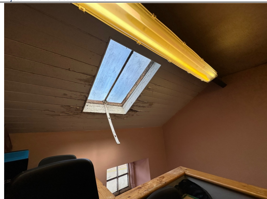
052 – General distortion in the alignment of the panel boarding to the sloping ceiling and a deterioration in the decorative finishes. Corrosion of the rooflight may be historical, but indicative that internal maintenance of this area has not been a priority. It is believed that issues with water ingress connected to the defective slate roof covering and also potentially the rooflight are contributing to the general deterioration of this area.
