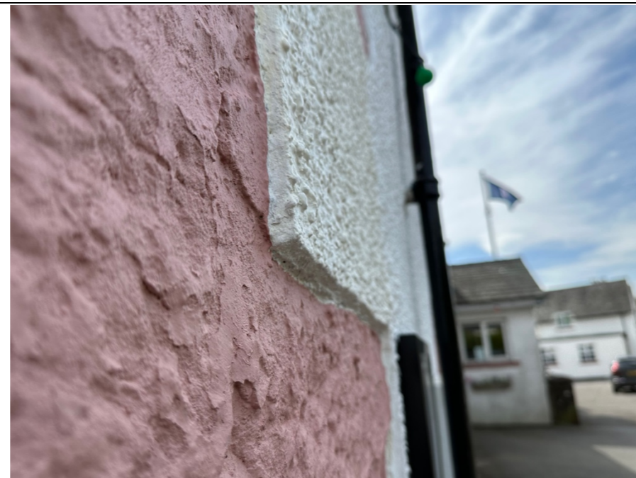
030 – A clear example of the incorrectly applied cement based rough cast render finish, which stands as much as 15mm in front of the original natural stone detailing.
