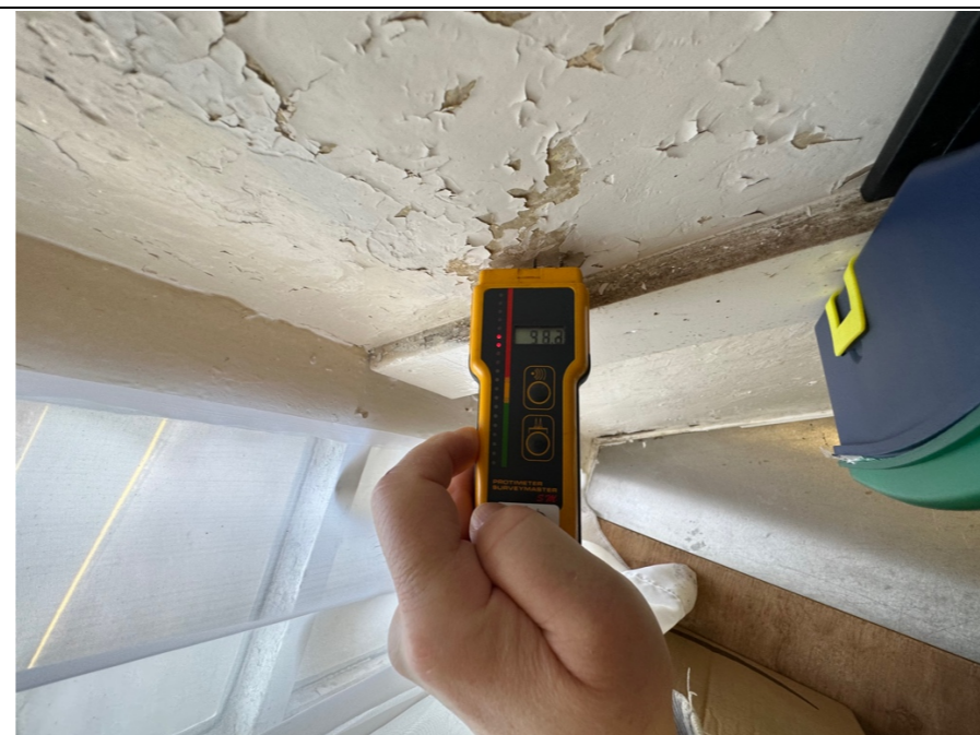
041 – Right hand internal wall reveal to the kitchen window, deteriorating condition of the decorated finishes, evidenced by the flaking paint finish.
