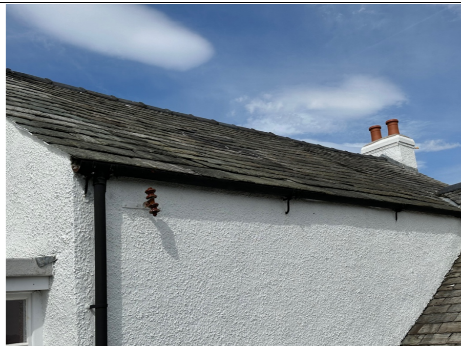
008 - South East facing slated pitched roof slope of the traditional Grade II Listed building.
