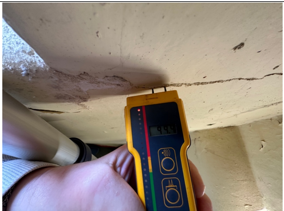
077 - Mid-level wall panel between at the sill level of the higher window. Evidence of localised movement and cracking in the gable wall at this location. Recommend monitoring of the crack using tell-tales and advising the buildings insurers that monitoring is being put in place. In this location the Protimeter presented moisture levels of 99.9%. Representing almost total saturation of the structure.
