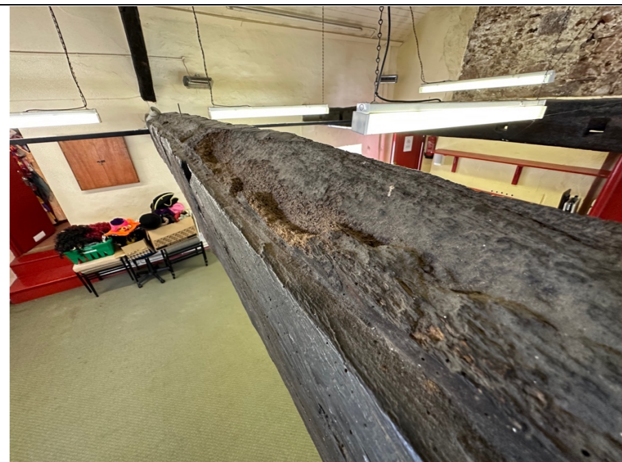
079 – Typical view across the upper surface of the bottom chord of a principal roof truss. Evidence of older wood boring insect activity.
