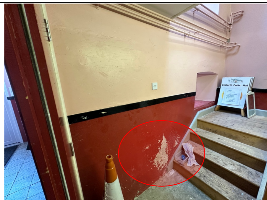
047 – Principal front wall of the traditional structure. Note: The deteriorating finishes at the base of the front wall.
