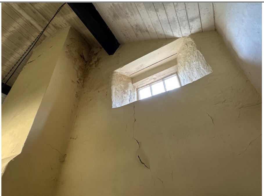
081 - General deterioration of wall finishes and boarded ceiling finishes to the right hand side of the chimney structure.
