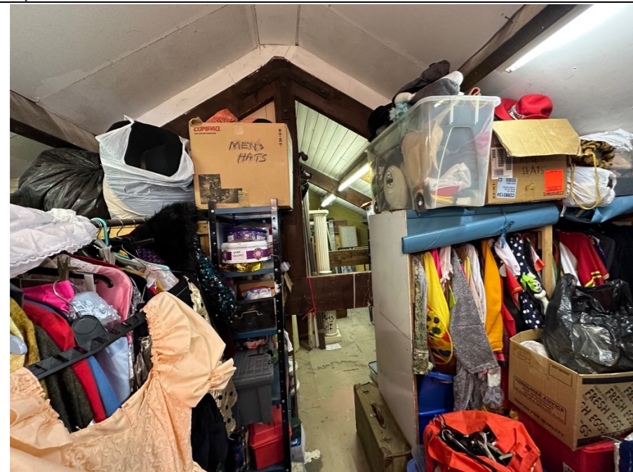
082 – General view of the store area above the Library within the two storey rear addition to the traditional building. Note the extensive loading up of the floor structure.
