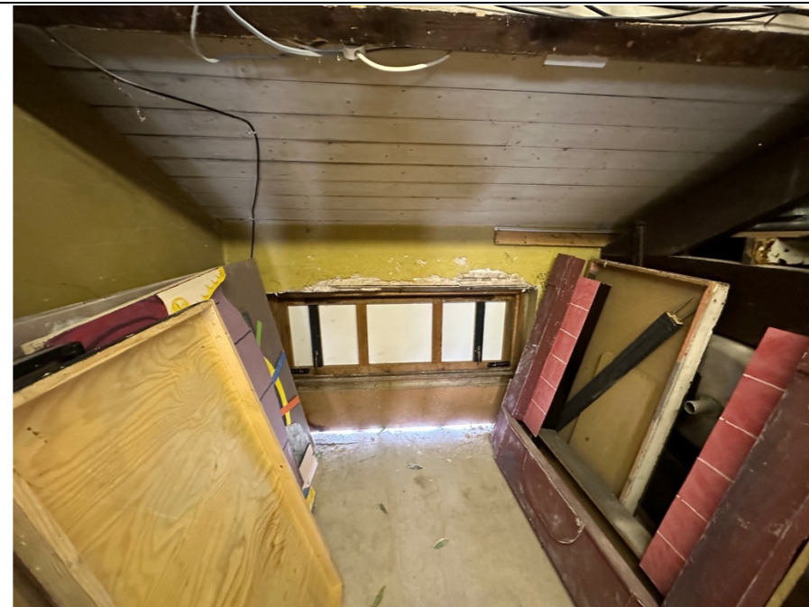
086 – View of the South West facing external opening within the store room that looks over the rear car park area. Note: Daylight is visible at the base of the opening, suggesting that this opening is not 100% watertight.
