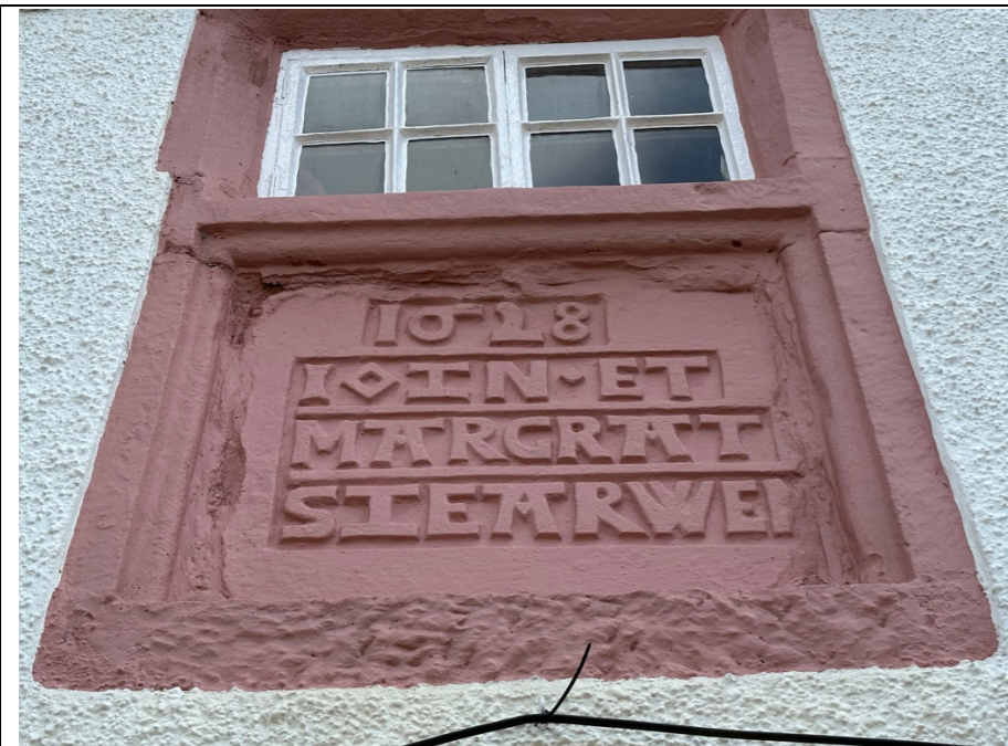
001 – Date of Grade II Listed traditional buildings construction. Original natural stone detailing painted over. Cement based rough cast render applied to all other masonry surfaces.
