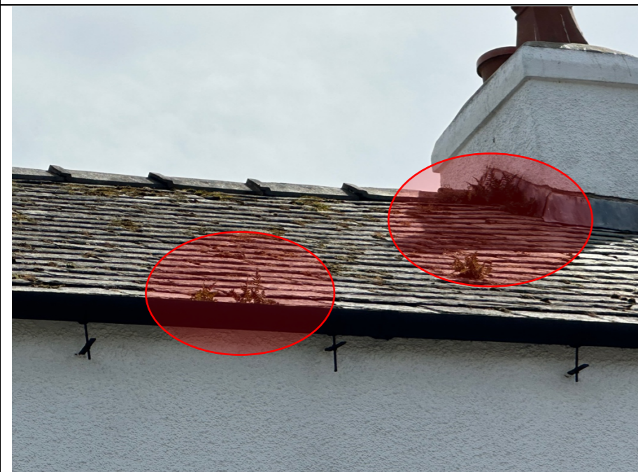
004 - Evidence of not just general moss growth to the pitched roof slated surface to the front elevation, but also of actual vegetation growing from beneath and between the slate roof covering. Indicated sufficient presence of damp to maintain vegetation growth. North West orientation.
