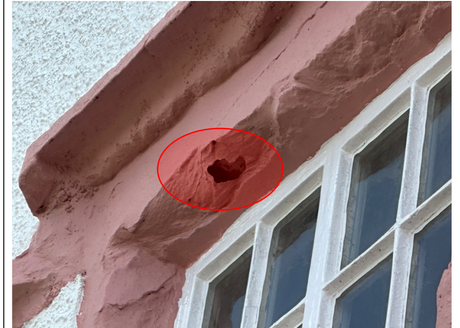
019 – The presence of the cement render will be contributing to the clear deterioration and general degradation of the natural stone mouldings to the elevation (typically sandstone). Despite being painted the stone detailing will be holding water which will be tracking through the stone, which consequentially will be causing the lamination of the stone and the break down of the painted surface finish.
