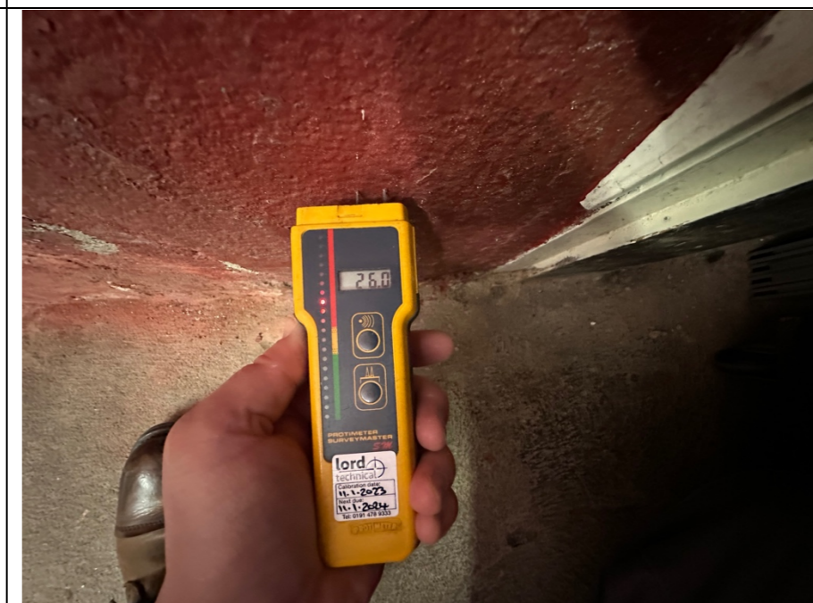
045 – Protimeter reading taken outside the internal store cupboard.
