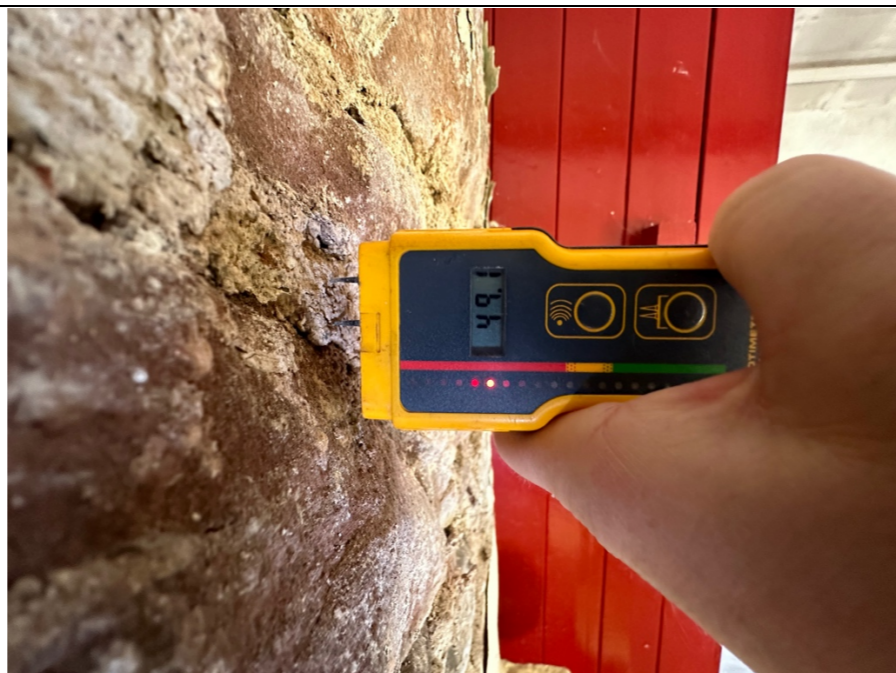
059 - Exposed masonry to the chimney breast structure identified in photo 056. In this location (chimney breast) the Protimeter presented moisture levels of 49.1%.
