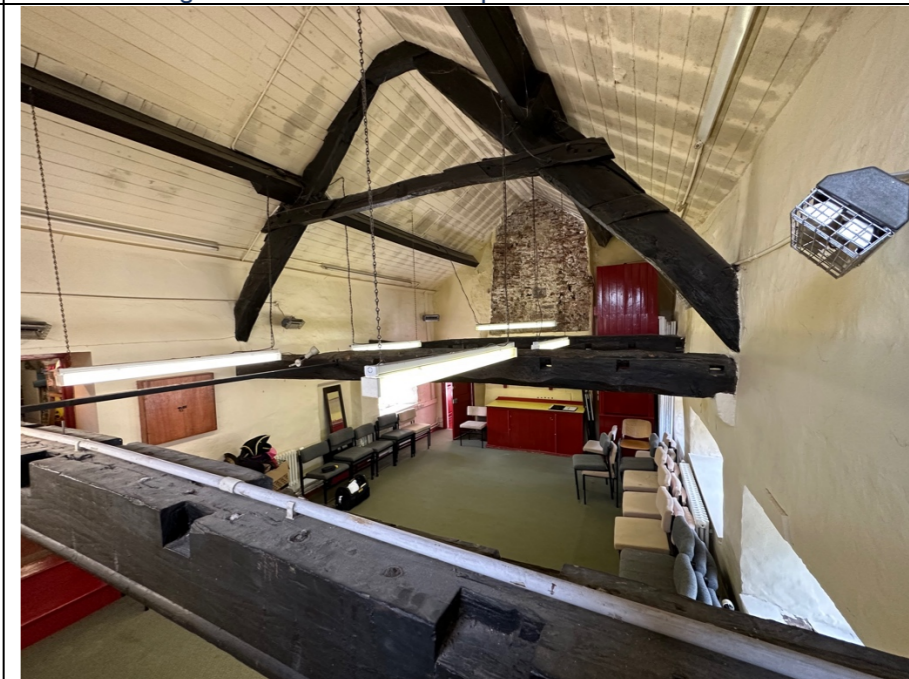
057 – General view of the first floor meeting room within the traditional constructed Listed building. Note the extensive discolouration to the timber panelling under-drawing the vaulted ceiling to the meeting room. This discolouration and marking is associated with the failing condition of the external slate roof covering and also indicates (as would be expected) a lack of insulation within the roof structure itself.
