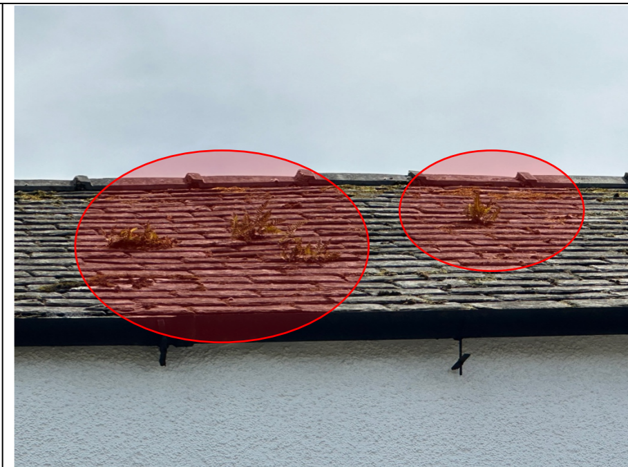
003 – Evidence of not just general moss growth to the pitched roof slated surface to the front elevation, but also of actual vegetation growing from beneath and between the slate roof covering. Indicated sufficient presence of damp to maintain vegetation growth. North West orientation.
