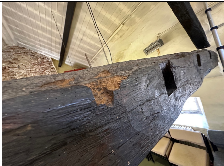
080 – Potential ongoing wood boring insect activity to principal roof trusses. Recommend inspection by an approved BWPDA technical representative to comment on status of noted damage to trusses.
