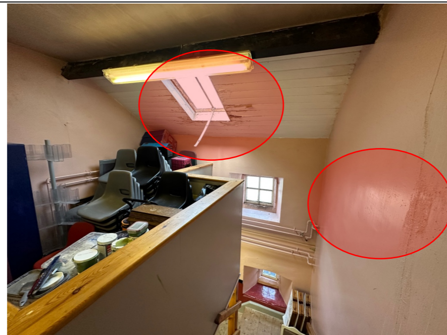
050 – General view of the first floor storage level, looking toward the front principal elevation. Note: Signs of water damage and deterioration of the panelled sloping ceiling area around the rooflight. Signs of water damage and surface disruption to the internal wall finishes, associated with water ingress (RHS of photo).
