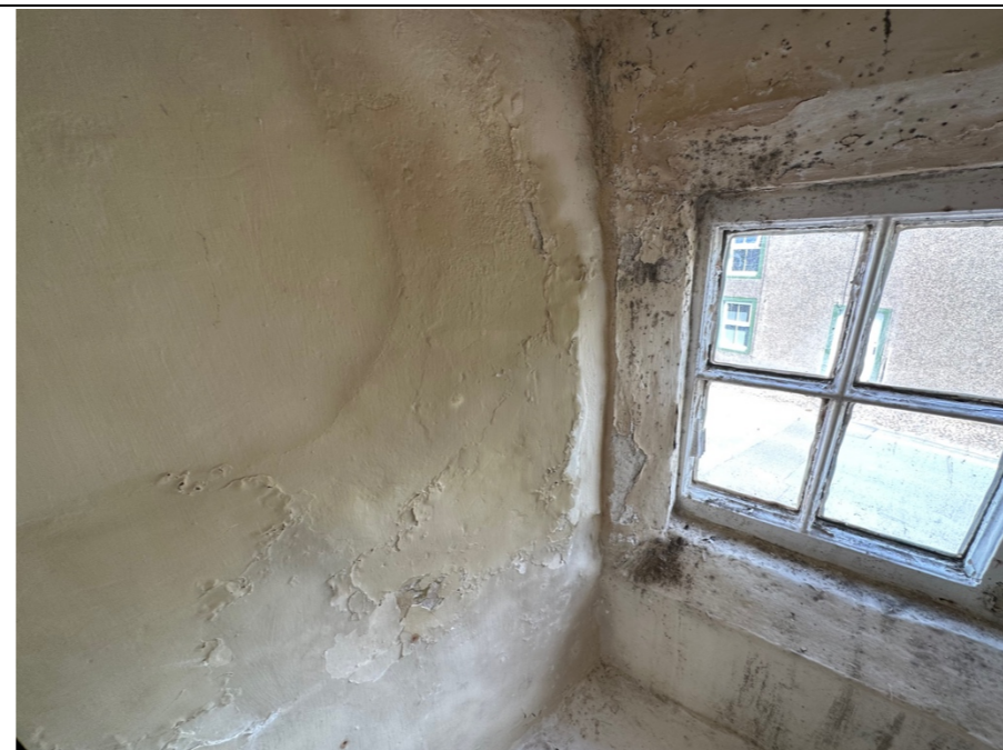
065 – Internal reveal of the window 01, extensive deterioration to both the internal wall finishes and the timber framed window joinery.
