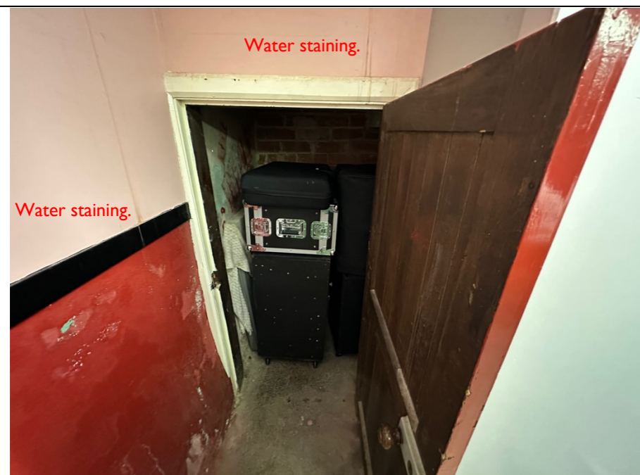
043 – Deteriorating and defective internal finishes to the internal partition walls, also presenting clear evidence of water ingress from higher levels as denoted by the water staining to the walls.
