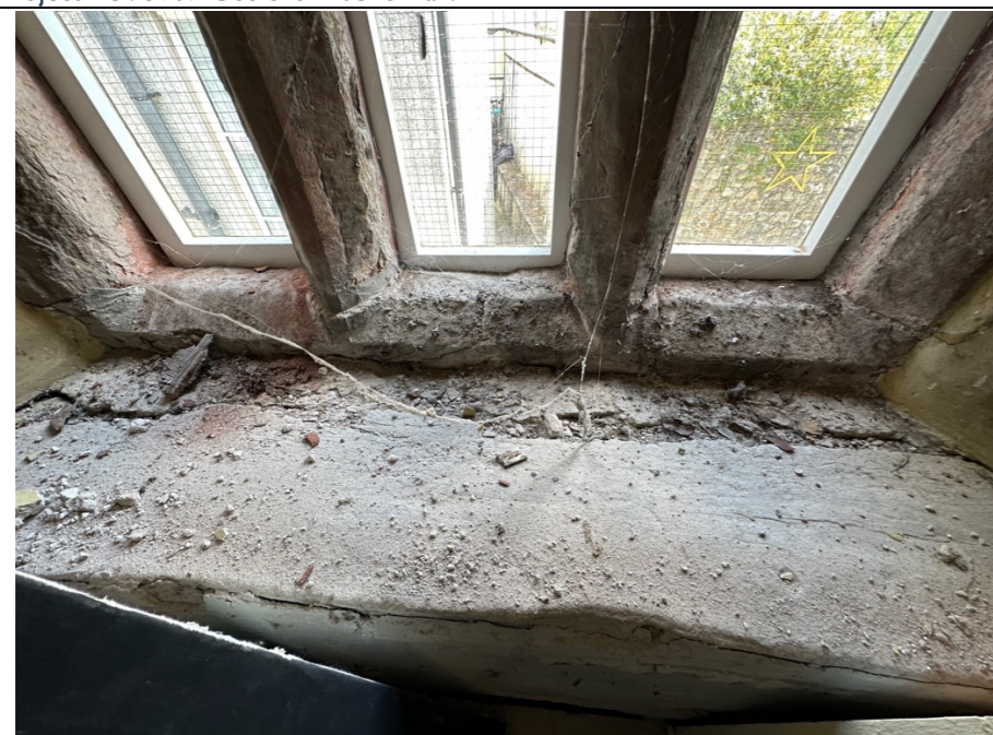
088 – Significant deterioration and degradation to the sandstone framing to the external window opening. Mullion sections are fractured and split.
