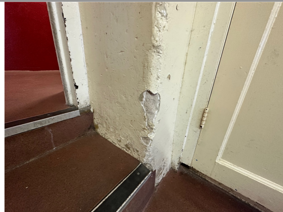
032 – Image of the door reveal between the rear corridor and the kitchen, illustrating the changes in level between the two areas.
