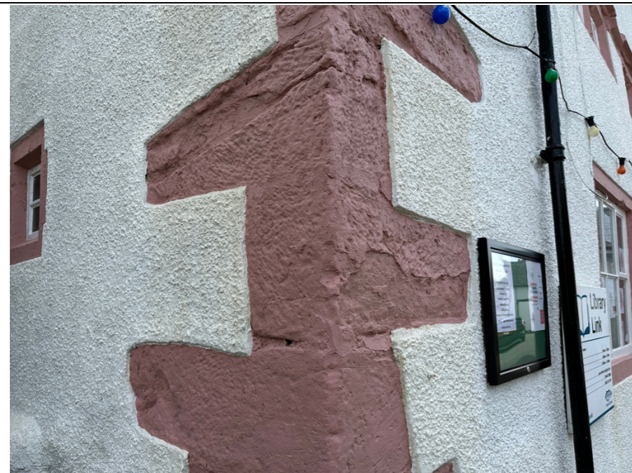
029 – As with the natural sandstone detailing external opening surrounds and the associated moulding details, the rough cast render finish has been applied / brought significantly forward of the natural stone.
