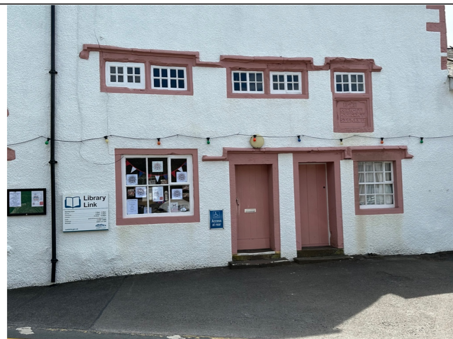
023 – General photo of the front elevation with clearer imagery of the areas of discoloured render associated with trapped moisture and water ingress behind the rendered surface.
