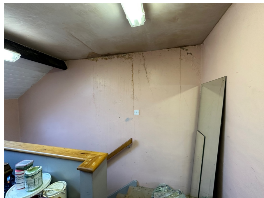
053 - Image of the recently plastered ceiling area above the staircase. Note: There is a discolouration and unevenness to the new plaster, indicative of the area retaining moisture and suggesting any repairs undertaken to resolve water ingressions have not been entirely successful. The tracking of running water down the internal face of the wall is also connected to the water ingression issues identified in photo's 043 – 046.
