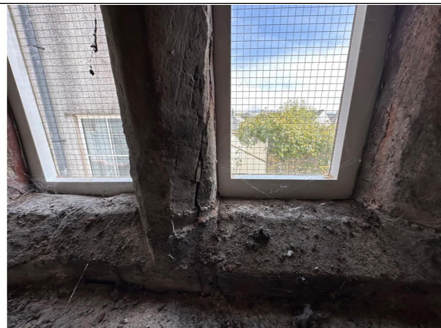
089 – Significant deterioration and degradation to the sandstone framing to the external window opening. Mullion sections are fractured and split.
