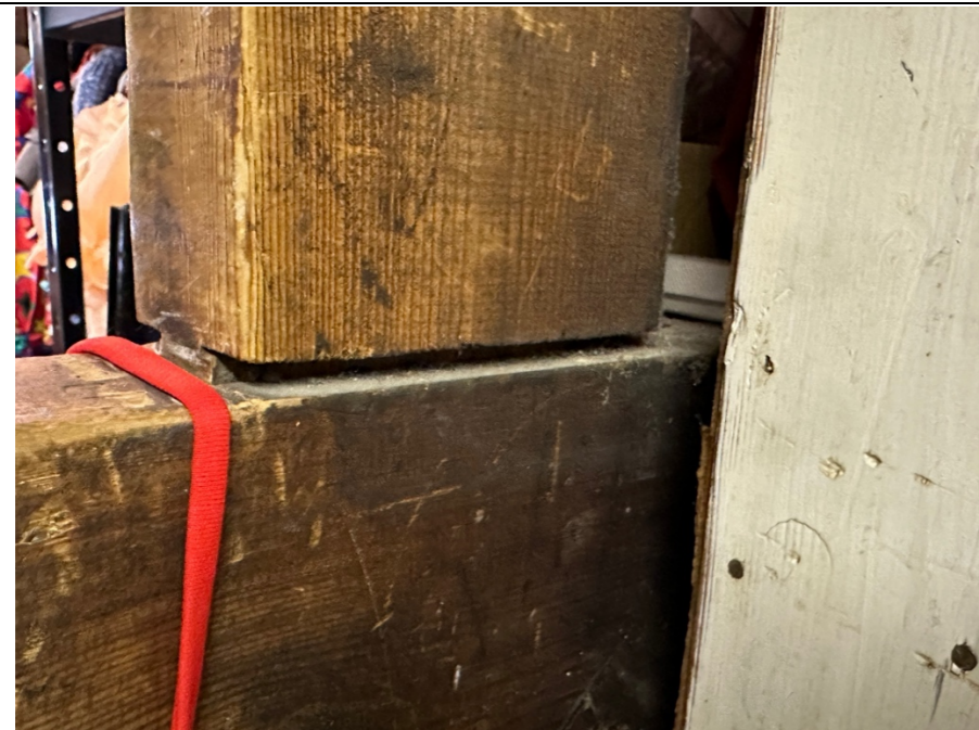
085 – A consequence of the additional loads imposed on the timber truss sections is that the joints between the truss members are being forced to part.
