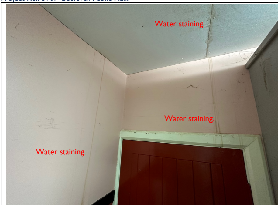
046 – View at a higher level of the door and associated walling / ceiling to the internal store cupboard ( refer to photo 043) with clearer evidence of the water staining and its affects on the wall and ceiling finishes. The unprepared finishes of the ceiling suggests that a repair has occurred in recent times, however the presence of the water staining would suggest that any repairs to resolve the issue with water leaks has been unsuccessful.
