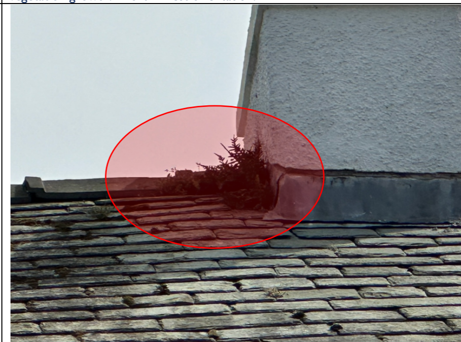
006 – During the survey we were advised that remedial works had been carried out to the external chimney stack to the South West facing wall of the traditional building. Whilst there is evidence to suggest that cement pointing repairs took place, it is clear the junction of the roof slate with the chimney stack is still holding water as proved by the vegetation growth at the junction.
