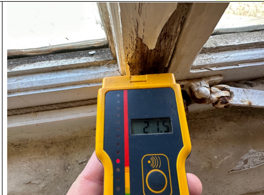
072 – Timber framing to principal elevation window. Complete breakdown and failure of the painted finishes to the framing.
