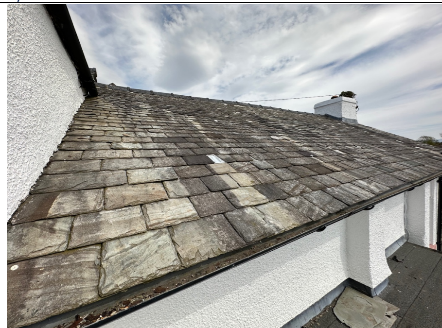
012 – General view of the South West facing slated roof slope to the rear addition of the traditional building. Note: The North East facing roof slope of the addition could not be viewed or surveyed due to access restrictions and difficulties getting a clear line of sight across the roof slope.
