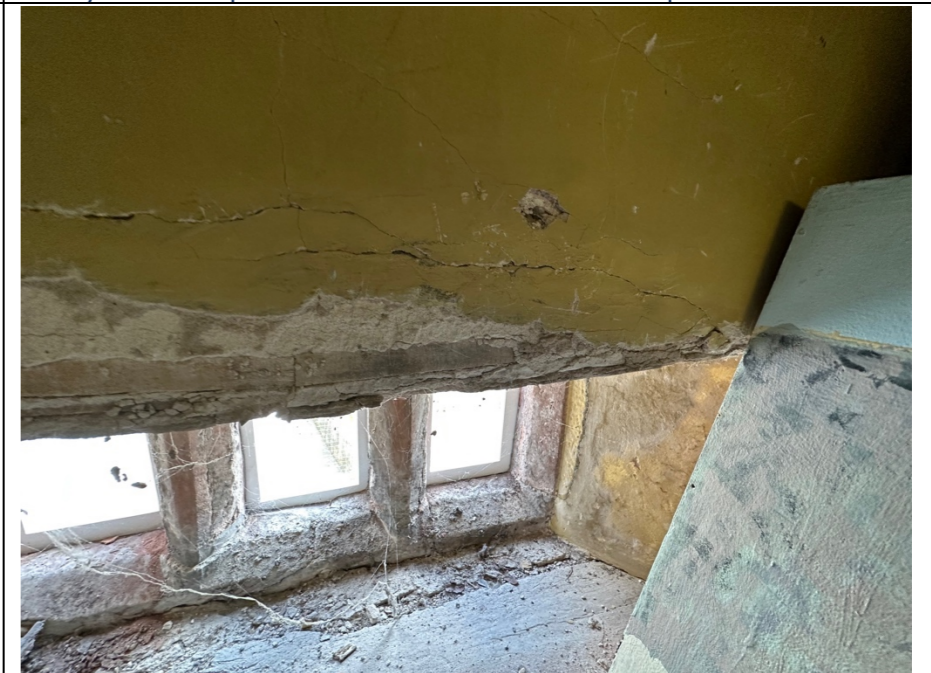
087 – Sandstone framed external window opening to the North East facing elevation. General deterioration of the lime plaster finishes, degradation to the sandstone framing.
