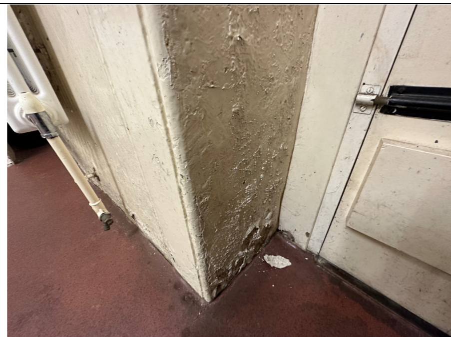
038 – Deteriorating painted (decorated) finishes to the internal wall surfaces to the front wall of the structure. Location, internal reveal to the external kitchen front door. Refer to photo 038.
