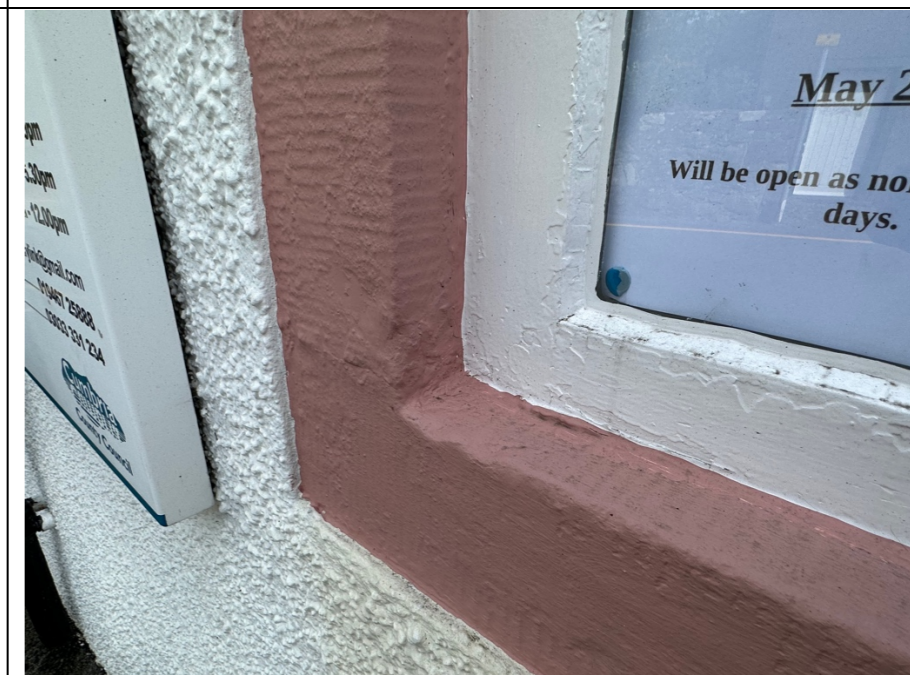
025 – Enlarged / close up image of the window opening and rendered finish identified in image 024.
