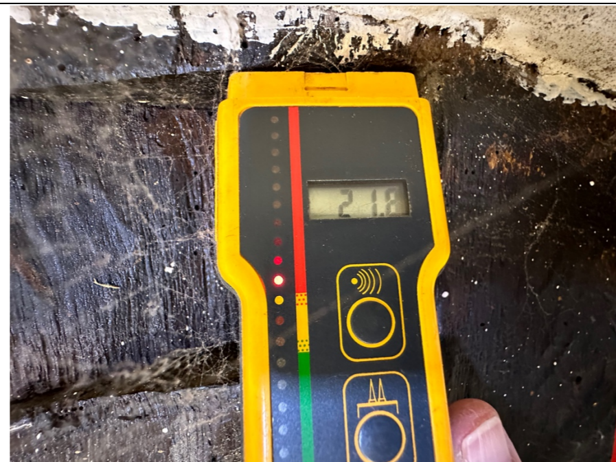
071 – Principal truss section identified in photo 070, protimeter recording the moisture level to the truss section itself within the meeting room.
