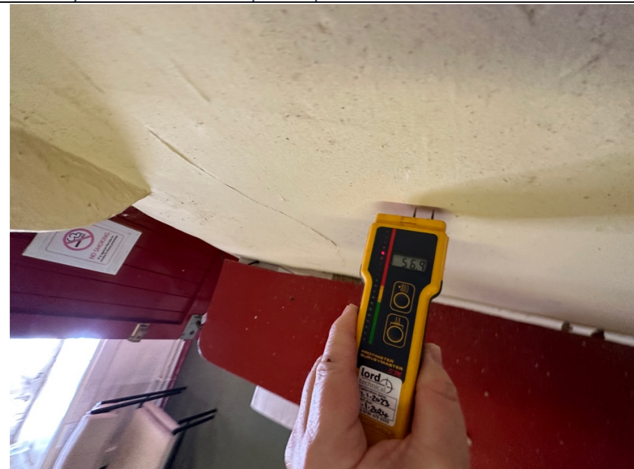
061 - Plastered masonry to the chimney breast structure identified in photo 056. In this location (chimney breast) the Protimeter presented moisture levels of 56.9%.
