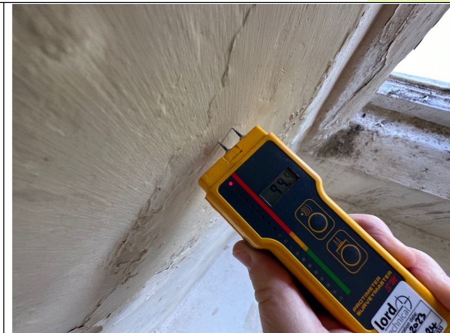
066 – Internal reveal of the window 01. In this location (window reveal) the Protimeter presented moisture levels of 99.9%.
