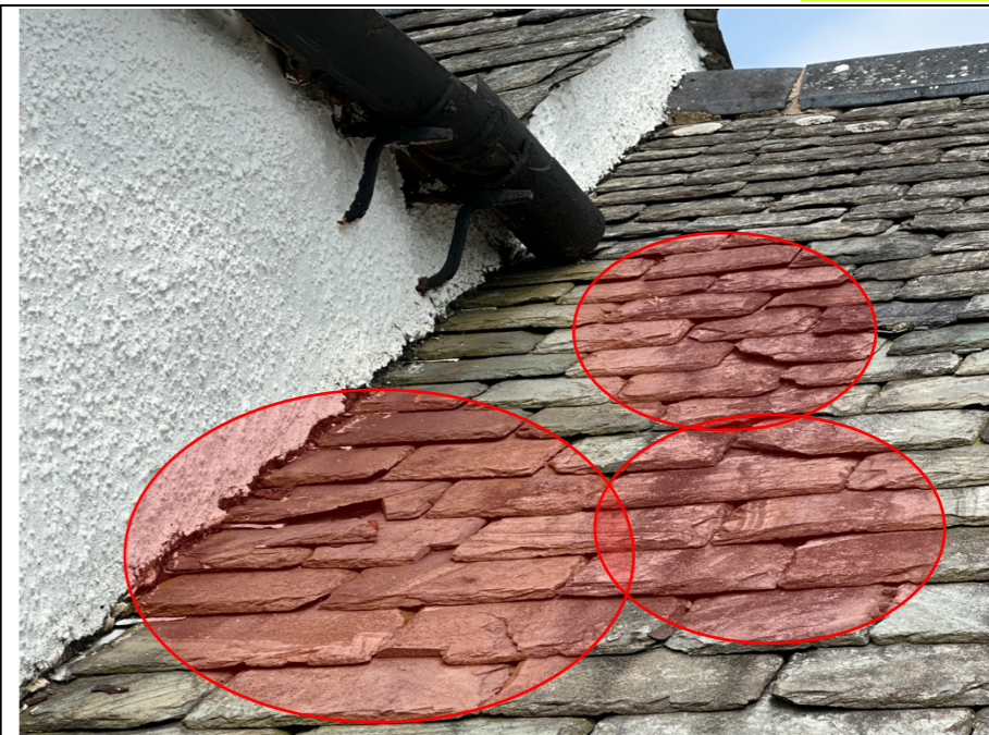
014 – Image taken of the rear addition slate roof area adjacent to the abutment with the Grade III Listed structure. Numerous examples of broken and damaged slates.
