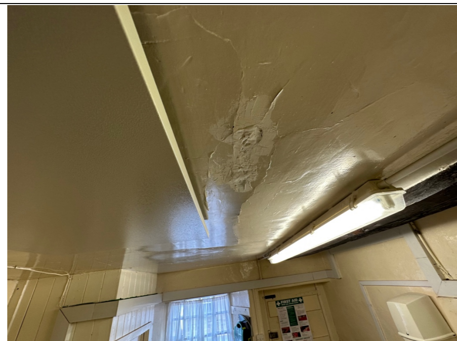
035 – Evidence of untidy and relatively unsuccessful previous repair attempts to the deteriorating kitchen lathe and plaster ceiling.
