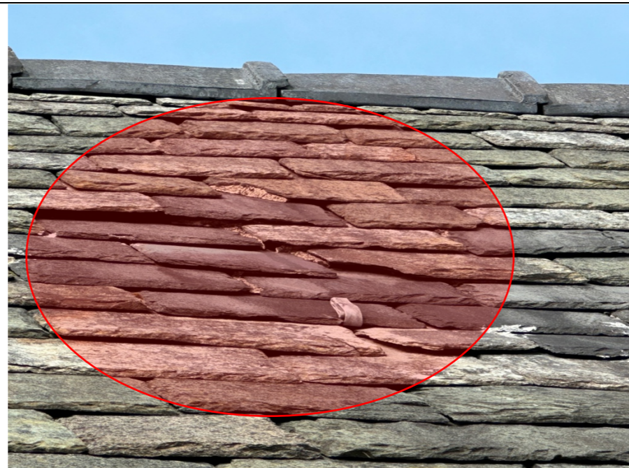
011 – South East facing roof slope, clear signs of lifting and gapping roof slate, broken slates and the use of lead tangles / tags to secure loose slates in place.
