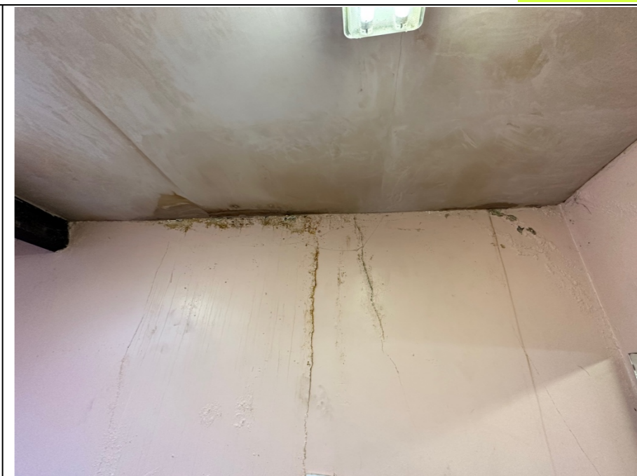
054 - Image of the recently plastered ceiling area above the staircase. Note: There is a discolouration and unevenness to the new plaster, indicative of the area retaining moisture and suggesting any repairs undertaken to resolve water ingressions have not been entirely successful. The tracking of running water down the internal face of the wall is also connected to the water ingression issues identified in photo's 043 – 046.
