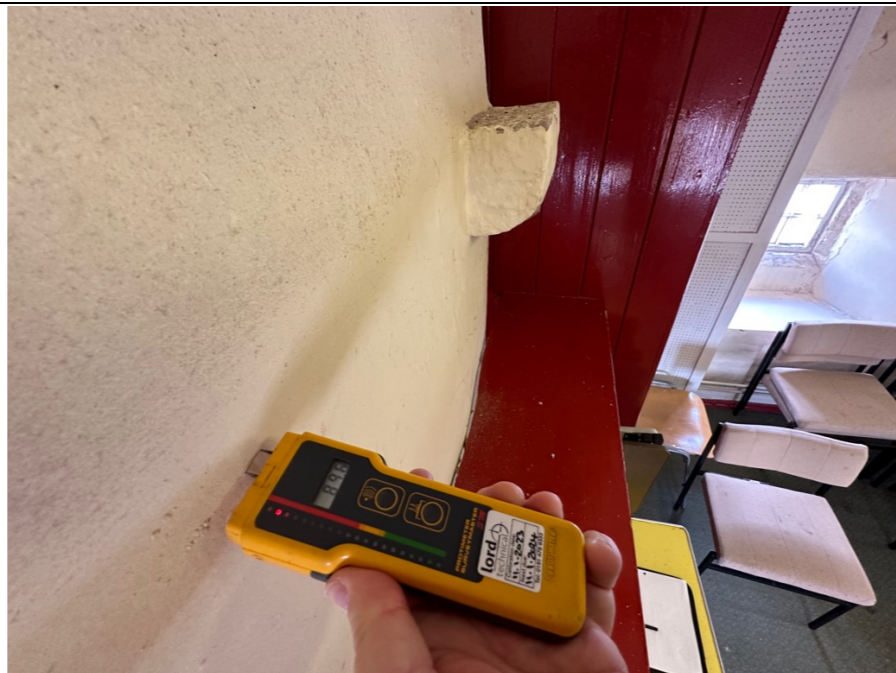
062 - In this location (chimney breast) the Protimeter presented moisture levels of 89.6%. Indicating almost full saturation of the structure.
