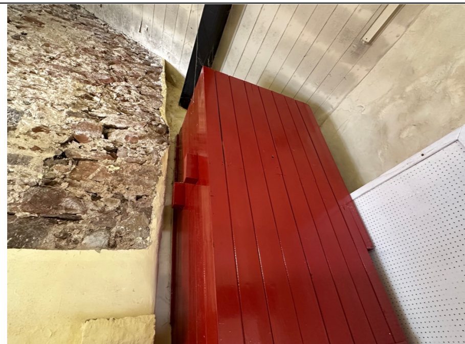
058 – Right hand side of exposed masonry to the chimney breast structure identified in photo 056. Note: Evidence of structural movement and bowing to the right hand side reveal of the structure. Recommend services of a structural engineer to inspect and report on any necessary remedial structural repairs required to stabilise structure.
