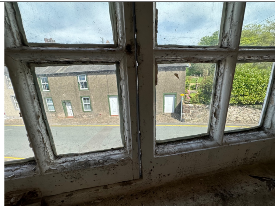
068 – Timber framed window in a poor decorative condition, evidencing of gapping between window components. All window joinery to this elevation is in need of an extensive overhaul and repairs.
