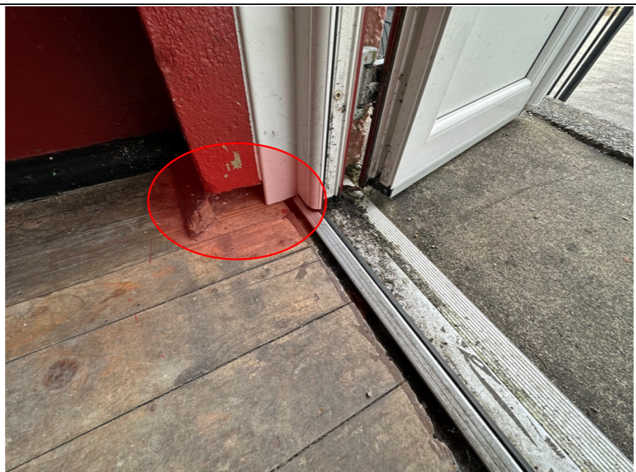
101 - Close up image of the issue noted in photo's 098 & 099. Note: the change in level and the evidence of the timber perimeter section parting company from the wall.
