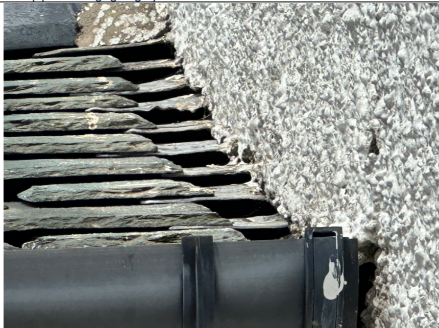
113 – Roof level view of the abutment between the lobby roof covering and the masonry wall to the Hall. Note: Gap of approximately 50mm between the slate edges and the rendered wall, exposing the lead soakers placed to help with weathering the junction at roof level between the two structures. At apex of the roof a cement fillet has previously been added to bridge the void created by the movement in the structures.
