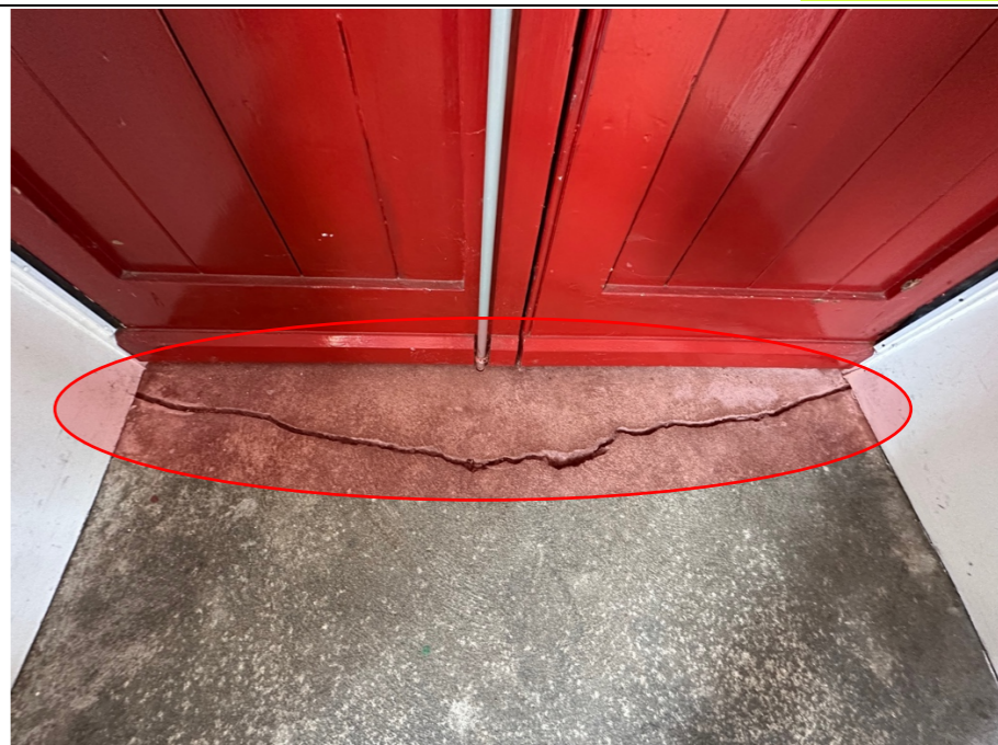
105 – Close up image of the defective floor structure identified in previous photos.
