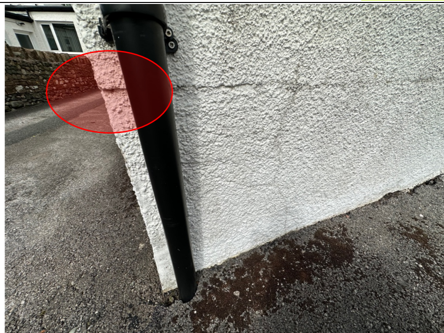
111 - Potential contributing cause for the noted movement in the lobby structure. Note: Horizontal line level with the top step of the structure and slight shift in the alignment of the structure external corner, alongside presence of a surface water downpipe discharging to gully.
