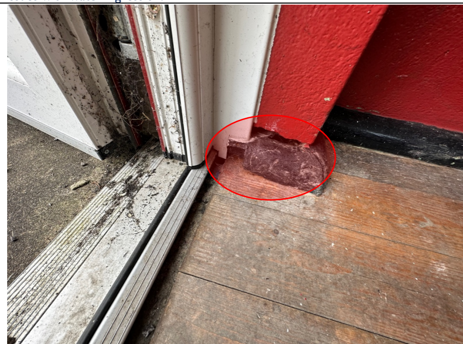
100 – Close up image of the issue noted in photo's 098 & 099. Note: the change in level and the evidence of the timber perimeter section parting company from the wall.
