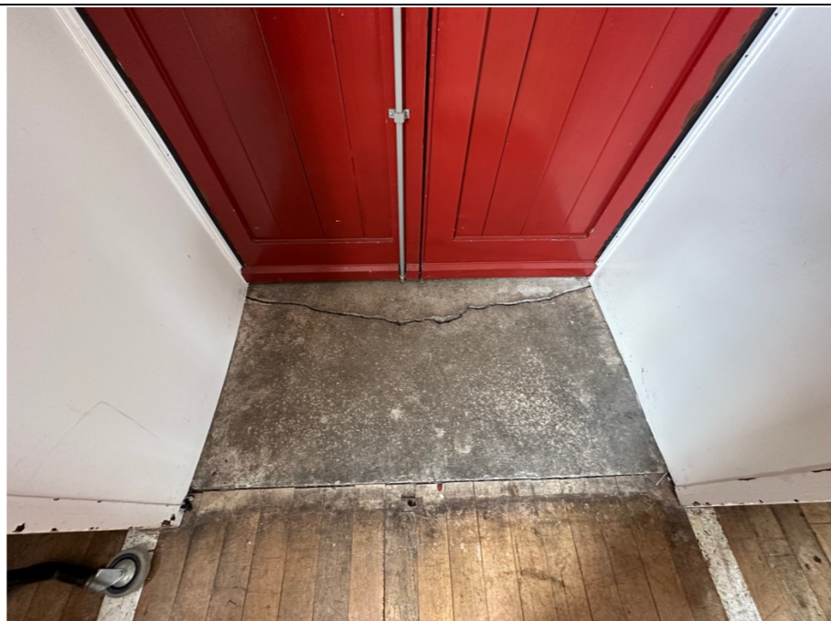
104 – Full width 'open' structural crack in the concrete floor structure to the entrance / exit lobby. Indicative of structural movement having occurred in this location.
