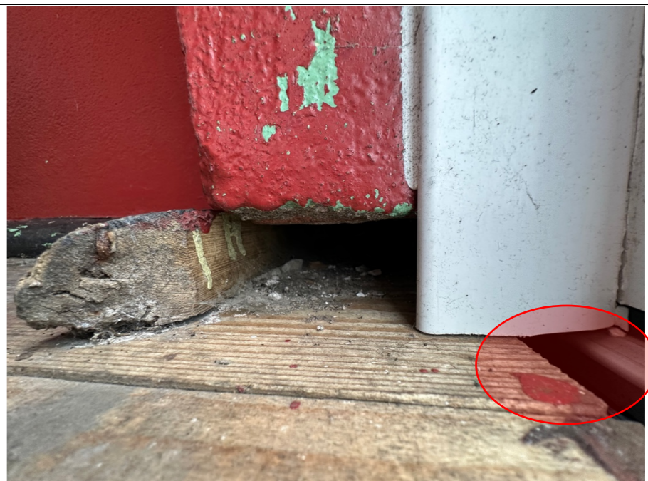
102 – Close up image of defective floor structure in the threshold area of the lobby entrance doors. Note: The timber flooring is not only dropping in level but pulling away from the aluminium threshold. Likely cause to be localised subsidence of the supporting sub-structure beneath the suspended floor or issues with water ingress and the rotting of the floor joist ends bearing into the masonry structure. Further destructive investigation recommended.
