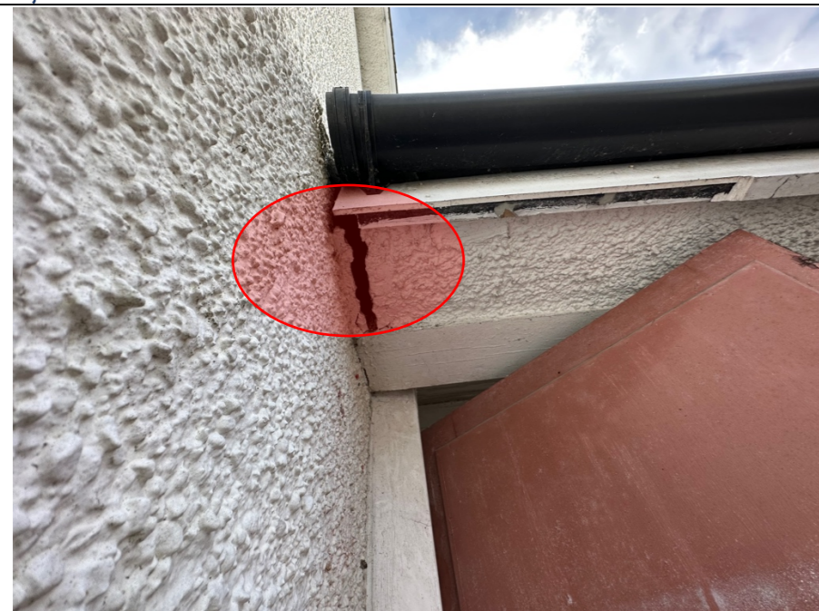
109 – External view of the entrance lobby, with clear evidence of movement in the structure away from the main building.
