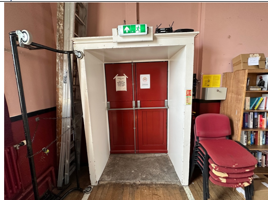
103 – Main Hall rear entrance / exit lobby. Cast concrete floor extending from suspended timber floor of the main hall.
