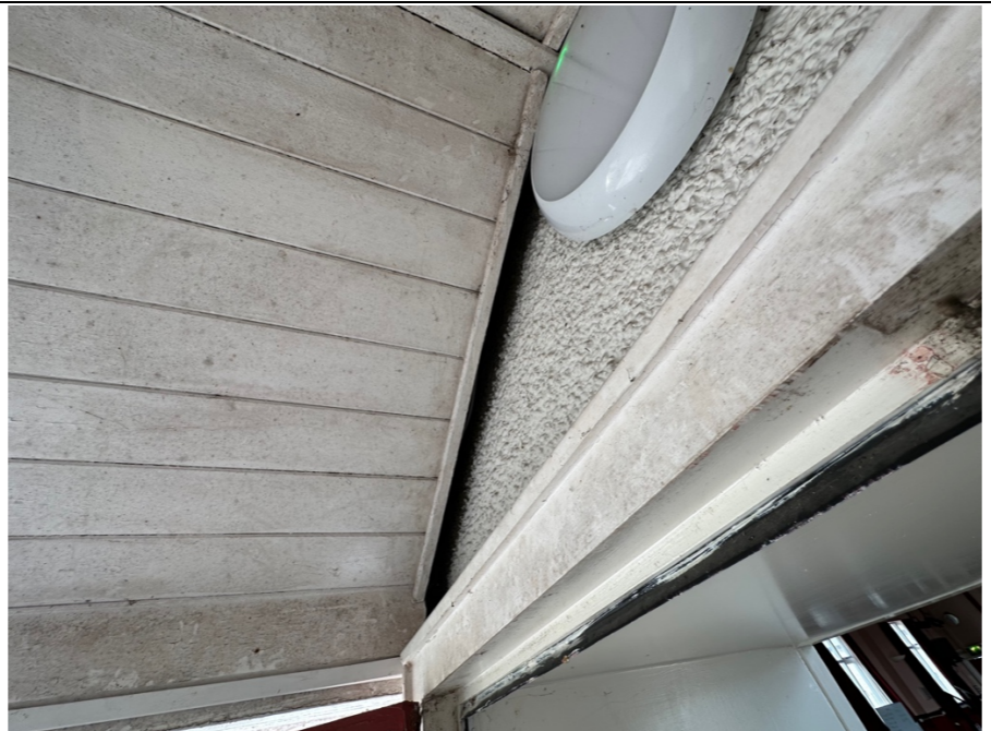
107 - View of the panelled ceiling structure within the lobby entrance (external). Note: Large void between the timber edge section to the ceiling panels and the rendered masonry wall.
