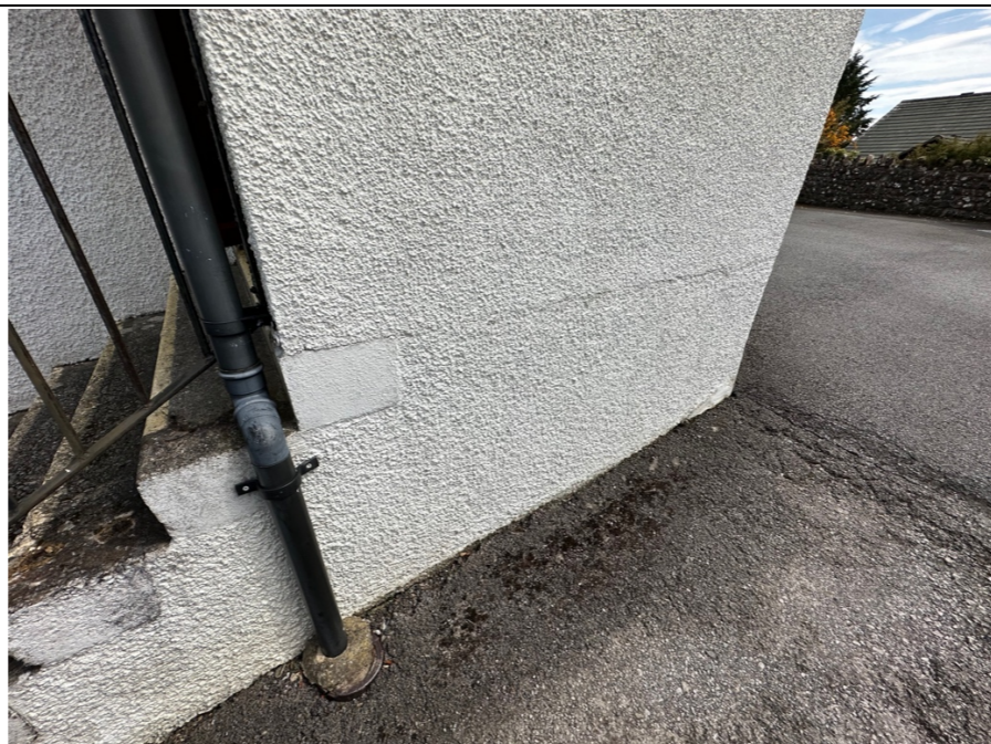
110 – Potential contributing cause for the noted movement in the lobby structure. Note: Horizontal line level with the top step of the structure and slight shift in the alignment of the structure external corner, alongside presence of a surface water downpipe discharging to gully.
