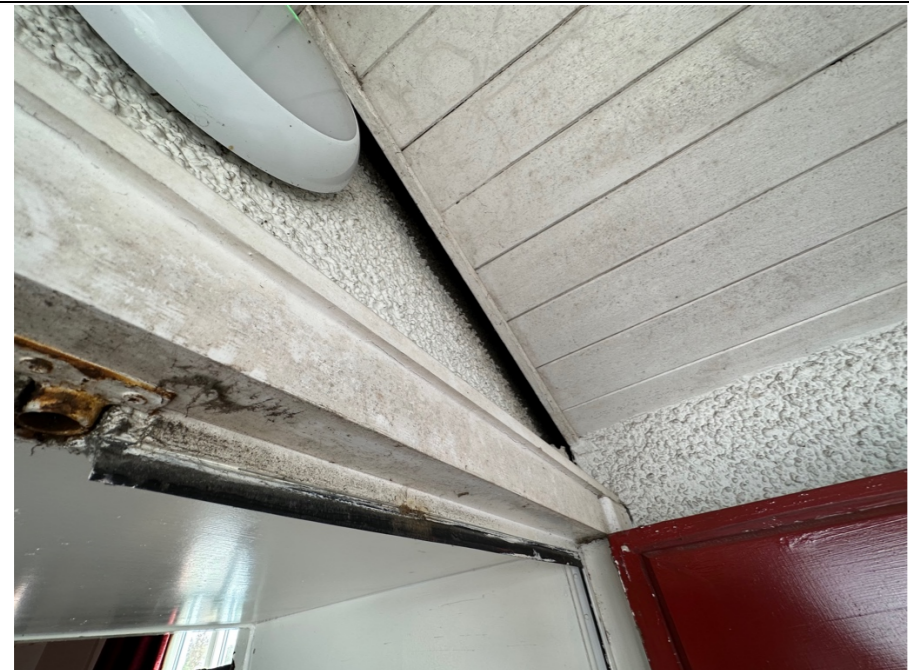
106 – View of the panelled ceiling structure within the lobby entrance (external). Note: Large void between the timber edge section to the ceiling panels and the rendered masonry wall.
