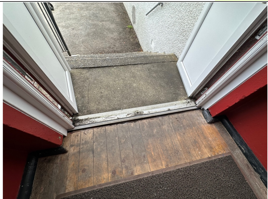
099 - Suspended timber floor structure to lobby with timber floor boarded finish. Note: General deflection and localised 'dropping' of the floor level across the width of the entrance doors.
