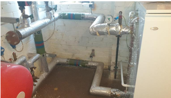
Oil Boiler & Header
