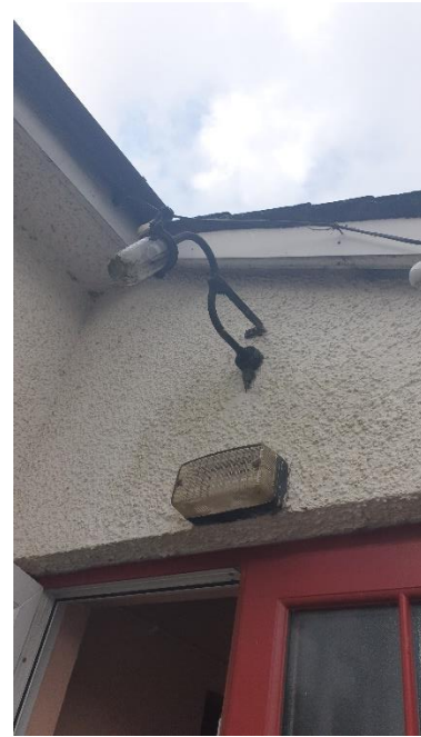
Basic External lighting.
