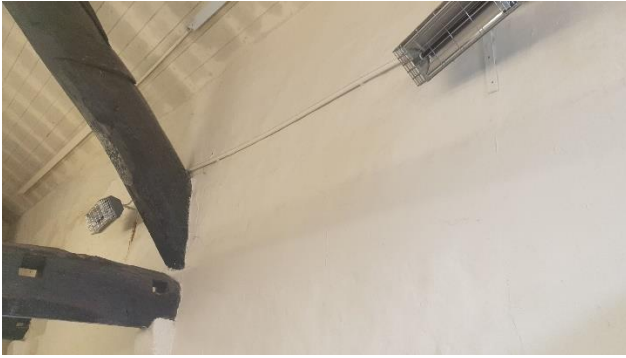
Infrared heater – Supper room
