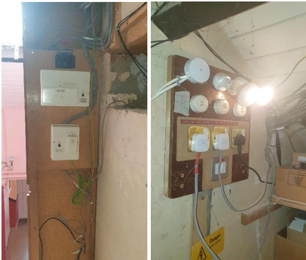
Older style rewirable fuses and Twin cable into plug tops
