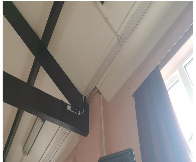
Extensions used in place of fixed wiring
