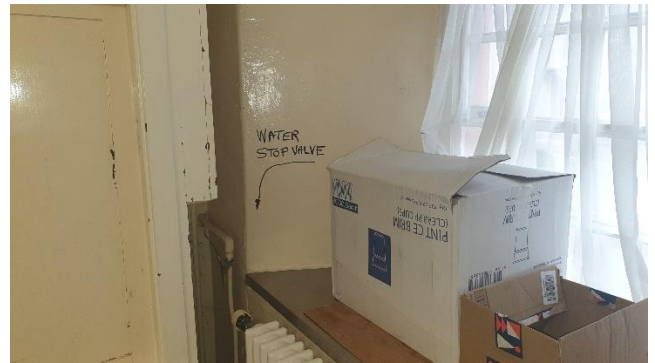
Incoming water supply - kitchen
