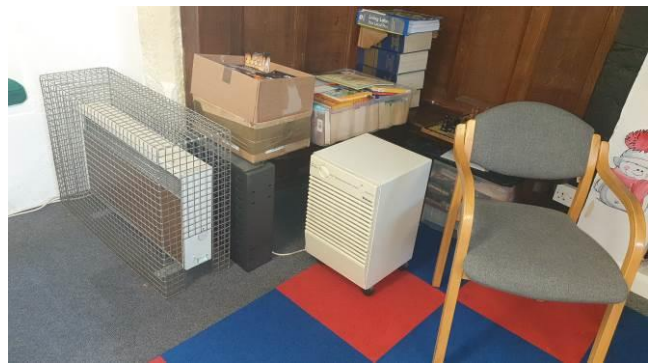
Electric storage heater
