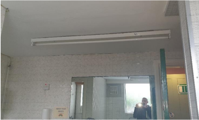
Exposed fitting in WC.
