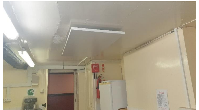
Radiant panel heater – kitchen
