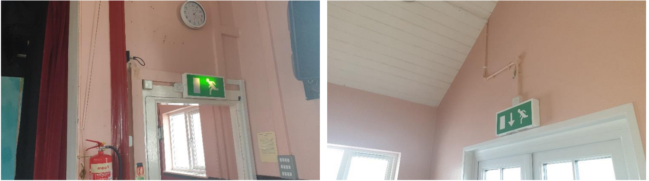
Existing Emergency Lighting
