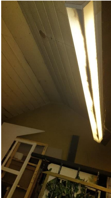
Luminaire in need of cleaning / replacement diffuser
