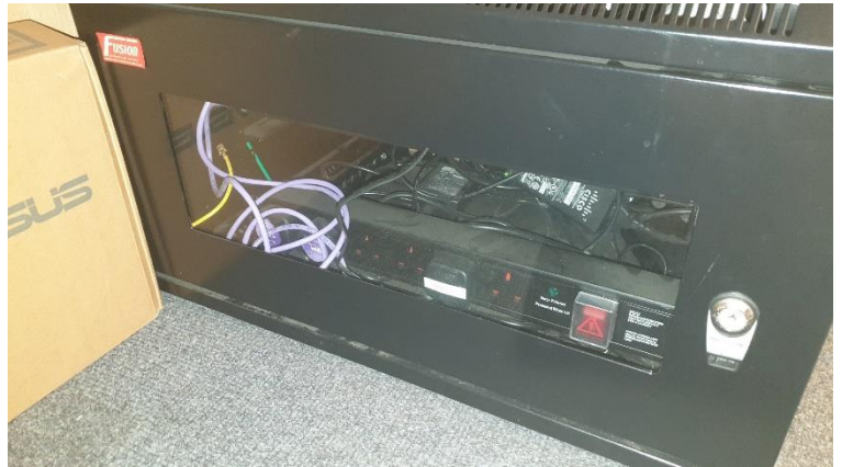
Data Hub located on floor
