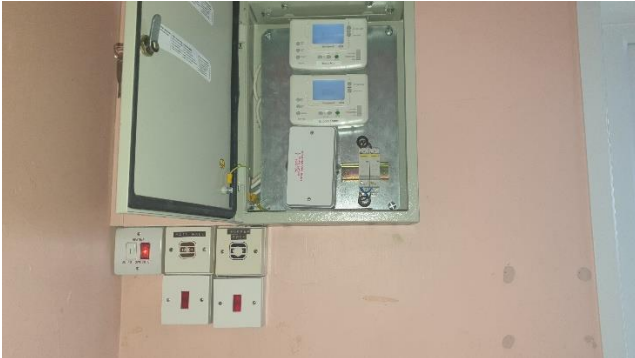
Heating controls and time extension switches
