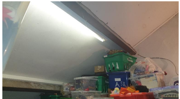
Exposed lamp fitting in store room
