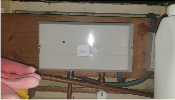
Instantaneous water heater – Kitchen
