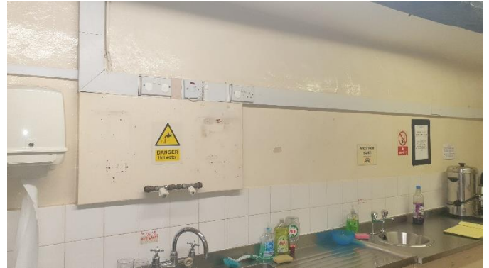
Location of old kitchen water heaters
