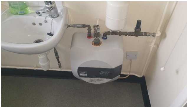
10 litre water heater – Disable WC
